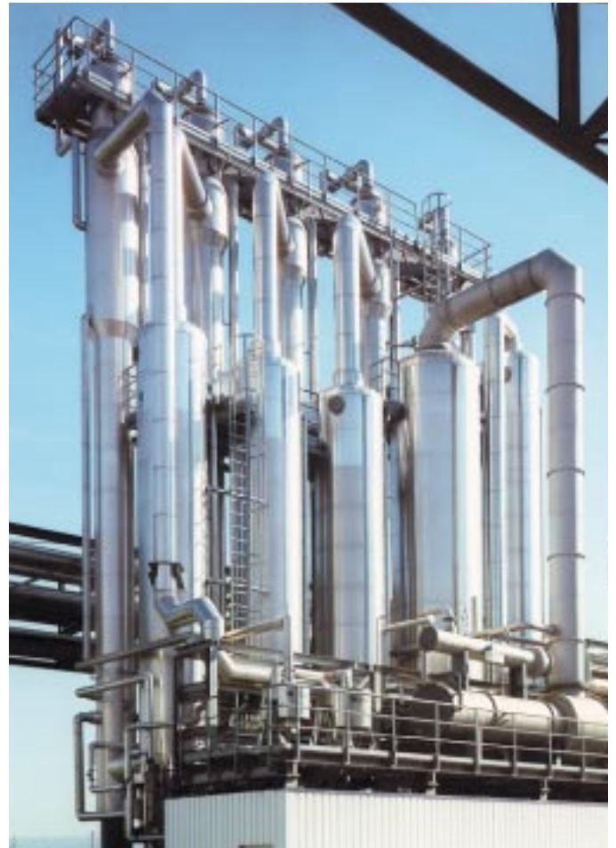
Right: A 4-effect, continuous rectification plant with falling film reboilers, downstream finisher and residue concentration system, designed for process water from the production of hollow fibre modules
